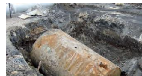
Figure 2 Discovery of buried chemical container
