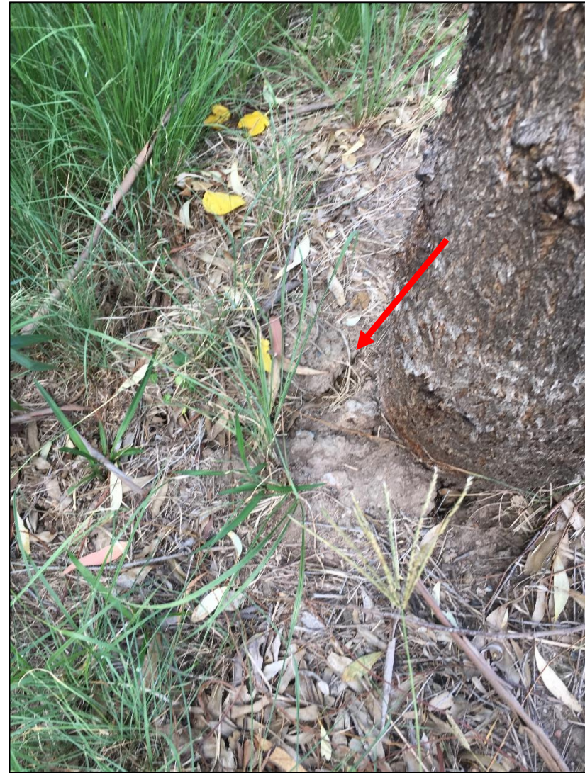
Plate 2 – Tree 196, appears to be moving in ground. Red arrow notes ground cracking.
