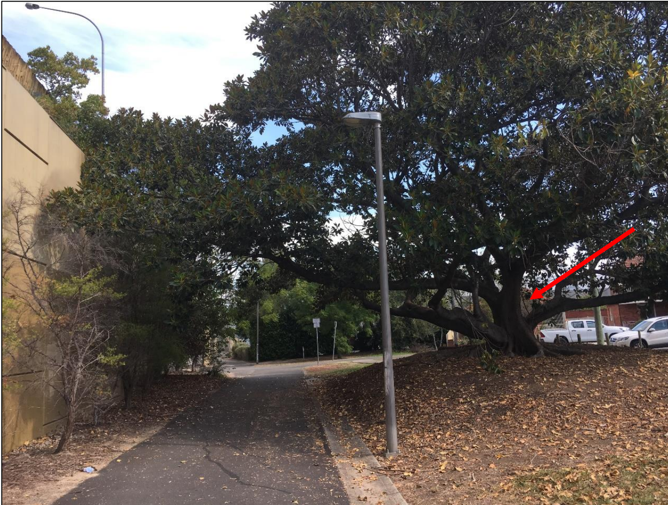
Plate 5 – Tree 76 noted with red arrow, is a significant tree and requires a large, low limb removed to accommodate access for equipment and excavation within the TPZ for sewer upgrade.
