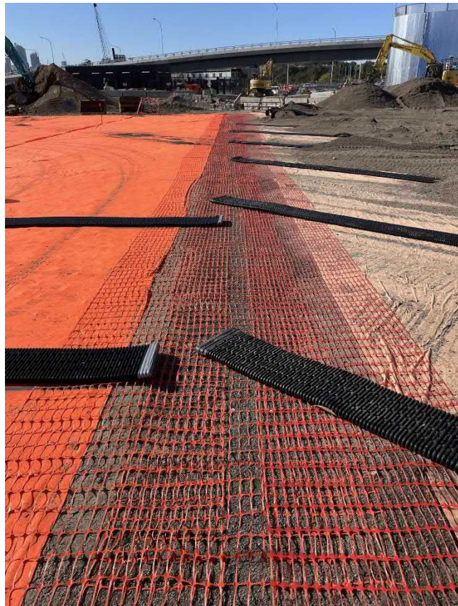
Figure 5.3 Mesh layer present at select locations beneath GC02 playing field
