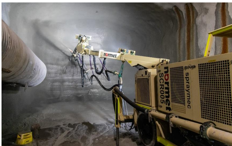
The tunnel roof being sprayed with concrete for ground support, also known as Shotcreting
