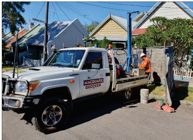
Example of a drill rig working in a local street to install ground monitoring equipment
