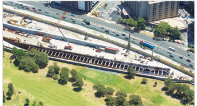
Ongoing excavation of the access decline where roadheaders will be deployed, February 2017
