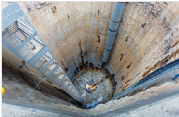
Crews have reached a depth of 40 metres in the tunnel shaft, February 2017
