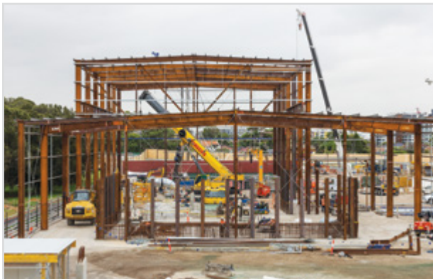
Construction of the steel frame for the spoil shed at Arncliffe, February 2017
