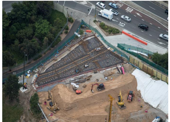
Aerial view of site preparation for the start of piling work at the Bexley south construction site, October 2016
