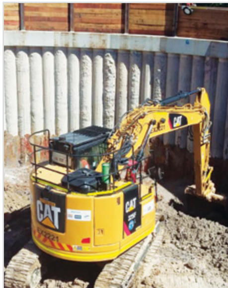
Excavation of the tunnel shaft at the Bexley Road south construction site, February 2017
