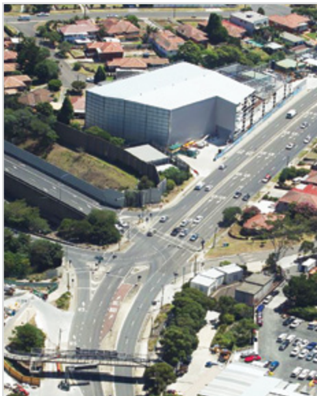
Construction of the acoustic and spoil shed at the Bexley Road north site nearing completion, February 2017
