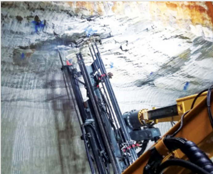
Drilling and installation of the roof support for the temporary access tunnel at the Bexley Road north site, February 2017
