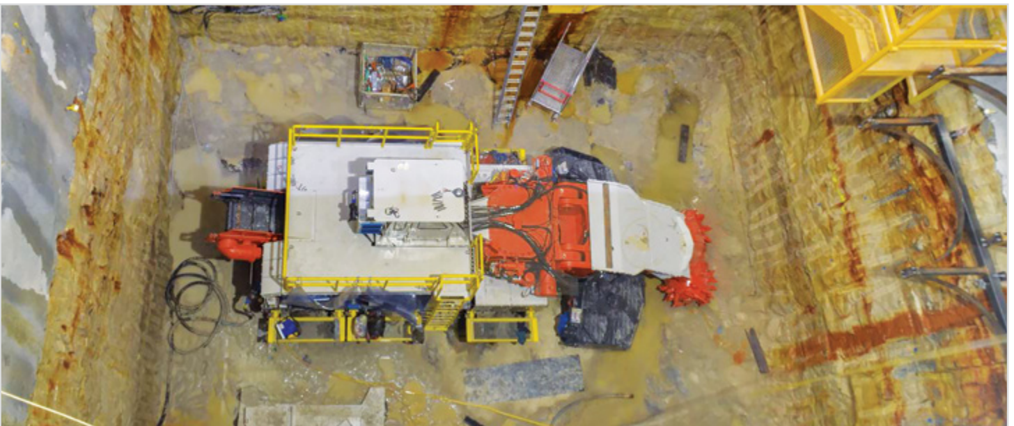
The first roadheader commenced tunnelling from the Bexley Road north construction site, February 2017
